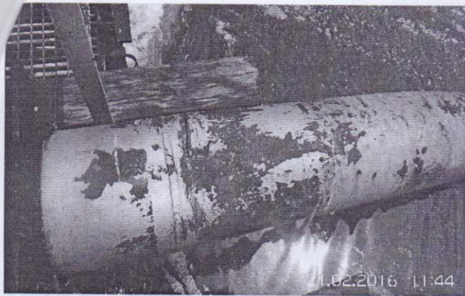
Figure 1: Hacksaw cut on a Riser.
